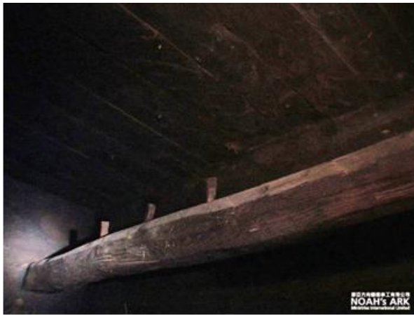
Is this a beam from Noah's Ark? Explorers with Noah's Ark Ministries International have released this photo of a wooden structure it says it has documented at an altitude of 13,000 feet on Mount Ararat in eastern Turkey.
